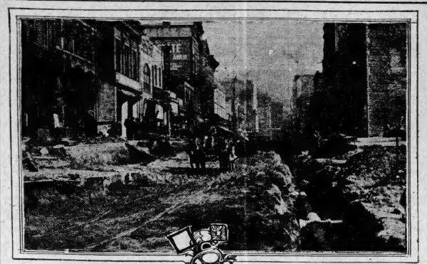
The illustration shows the county force at work on the new Whitehall street grade from Mitchell to Brewster streets.
